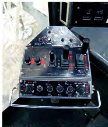
Tilt-type control panel
